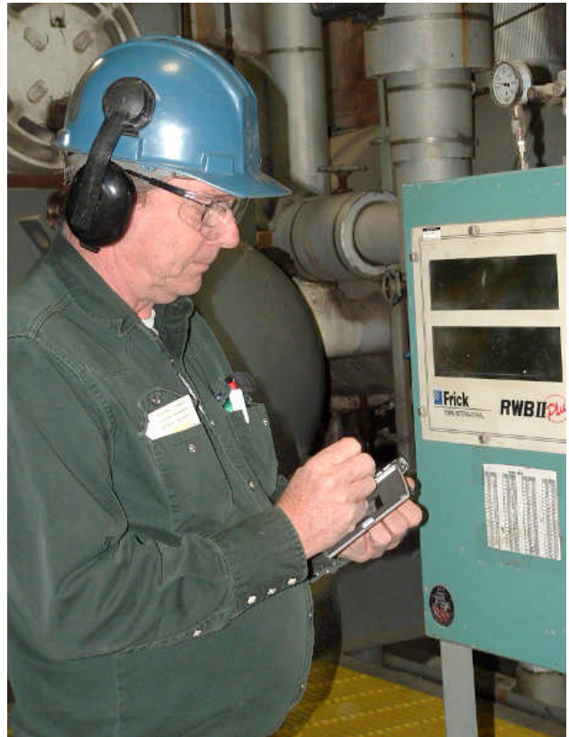
William Grippin Jr., a plant technician with Air Liquide, enters process data into a PDA using QWPocketPC
